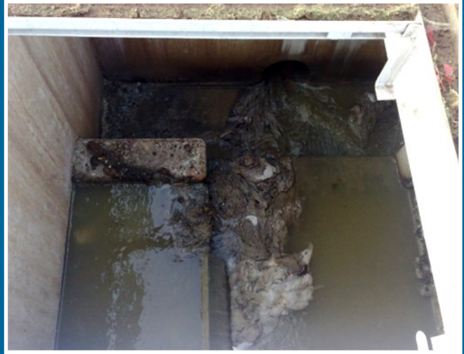
Figure 1: CSO spilling litter due to blocked screen
